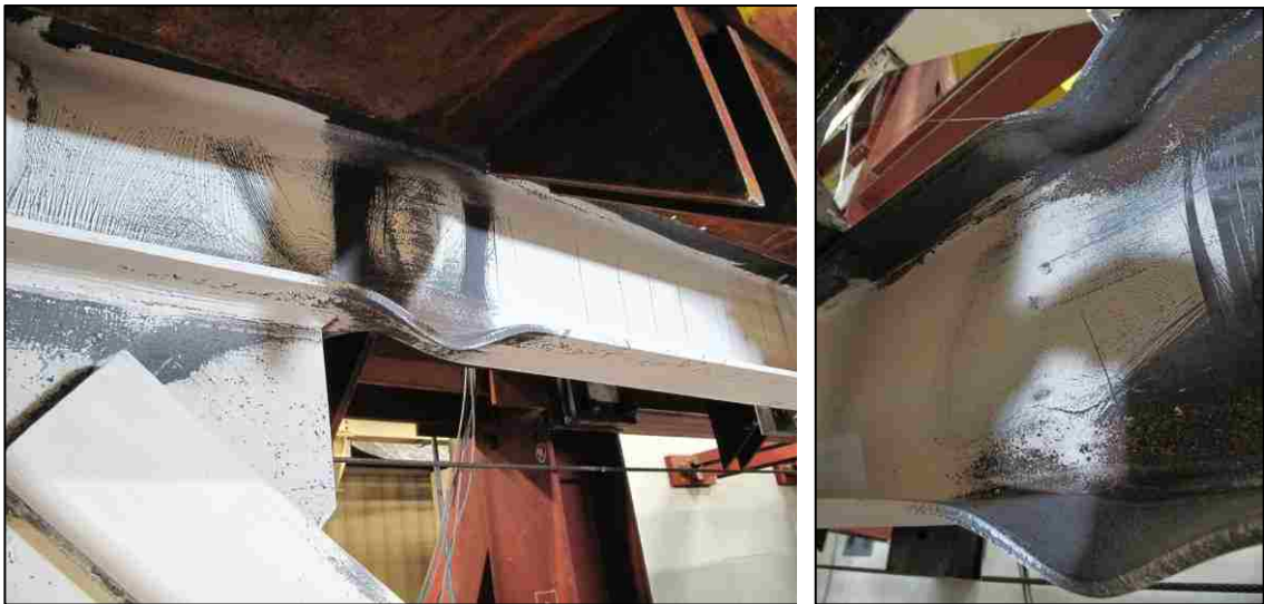
Figure 4.24 Local buckling in beam plastic hinge observed in Bradley et al. (2015)
